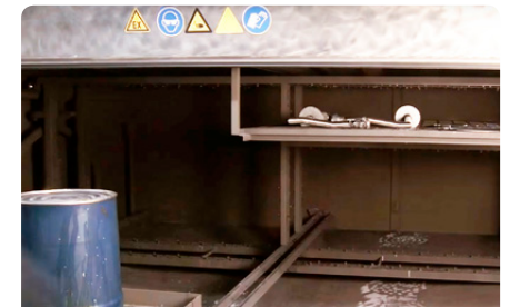
Fixed 2 nd Storey + Rotating Nozzles for Cleaning of Buckets
